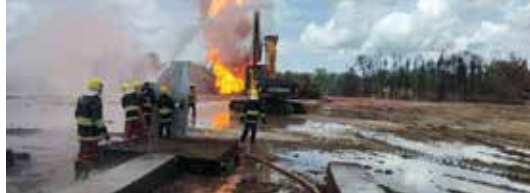
OIL Fire Service personnel assisting Alert and ONGC CMT team while working near well plinth by continuous spraying water jacketing the site
