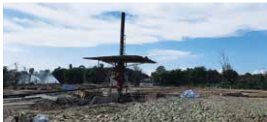
Baghjan well no 5 after diversion of flow of gas to nearby Early Production Setup (EPS) on 13th Sept 2020
